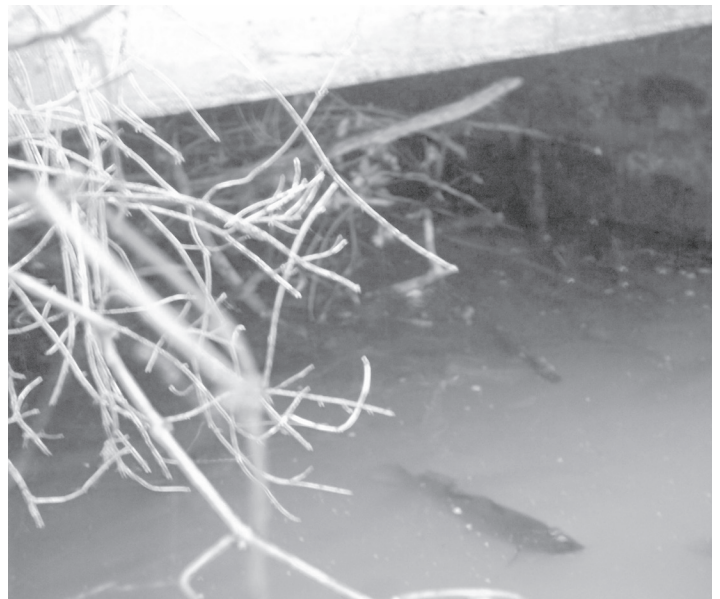
Figure 3. Debris dam (in background) within culvert.
